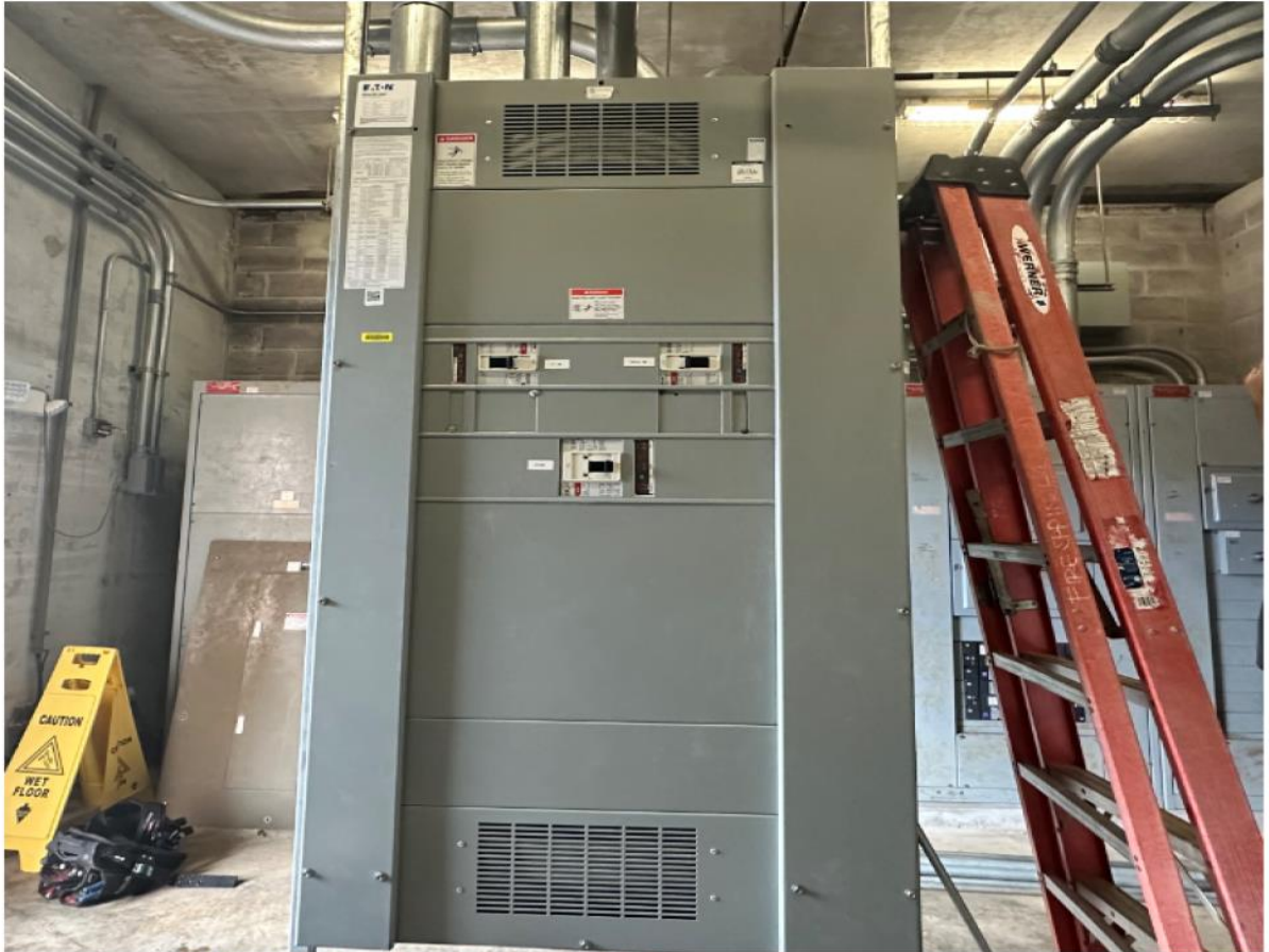
Figure 4: Existing Switchboard H / Transfer Switch
